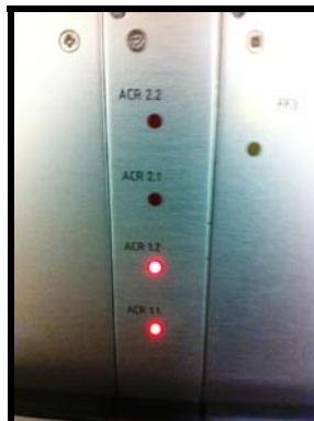
Fig. 23: AK19 module assigned to one Binary Counter Module with channels 1.1 and 1.2 activated. Both LEDs within the pair should illuminate when the ACR key is actuated.
