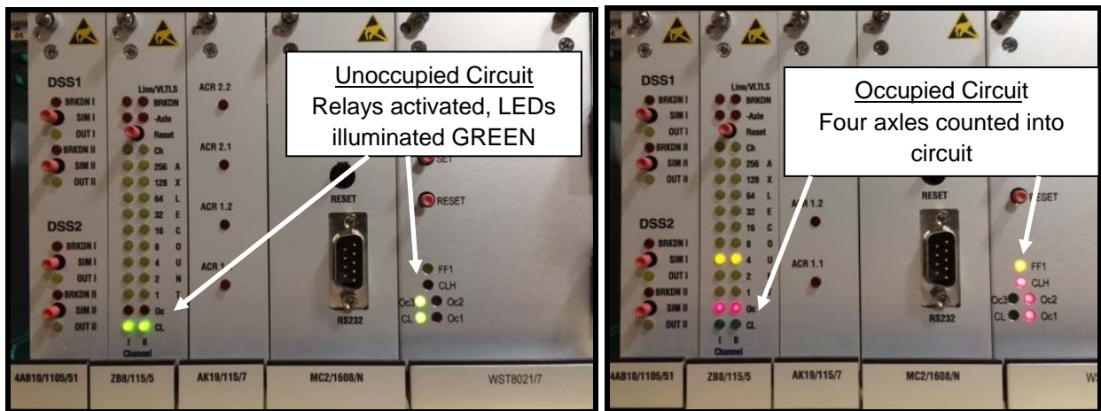
Fig. 19: LED indications (counter module and clear signal relay module) for clear and occupied axle counter circuit status
