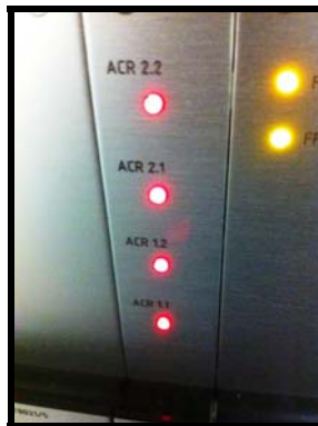
Fig. 22: AK19 Module assigned to two Binary Counter Modules with four channels in use. Red LEDs should illuminate when the ACR key is actuated.
