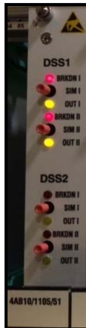
Fig. 12: Amplifier card front panel indicating DSS off-rail condition. Note both yellow “OUT” and red “BKN” LEDs illuminated.
