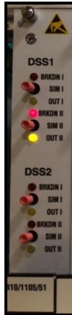
Fig. 13: Amplifier module front panel indicating DSS 1 SII shorted or open cable. Note both yellow “OUT” and red “BKN” LEDs illuminated.
