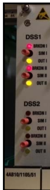
Fig. 14: Amplifier module front panel indicating DSS off-rail condition. Note both yellow “OUT” and red “BKN” LEDs illuminated.
