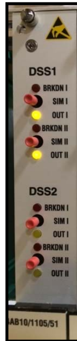
Fig.15: Metallic Object or Wheel Flange Resting Atop Both Systems of the Sensor
