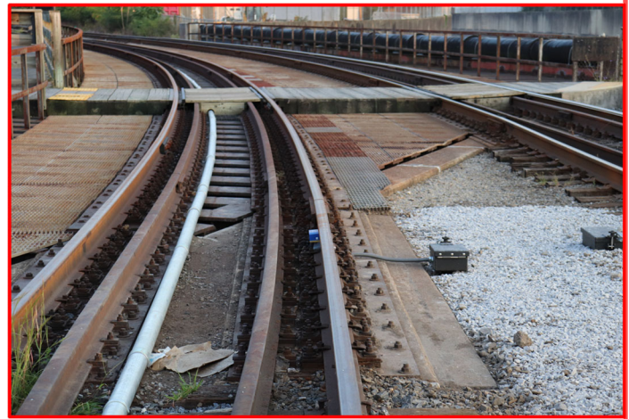
An axle counting system provides the needed reliability where a steel-deck bridge extends into the approach of a highway grade crossing system.
